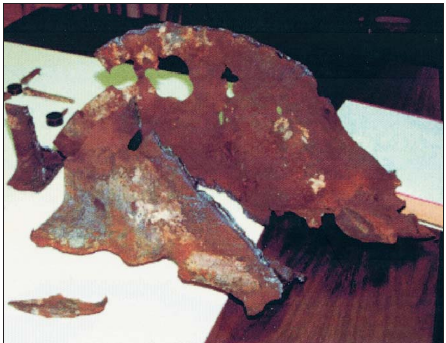
Figure C-1 Eroded A36 wide-flange beam.
