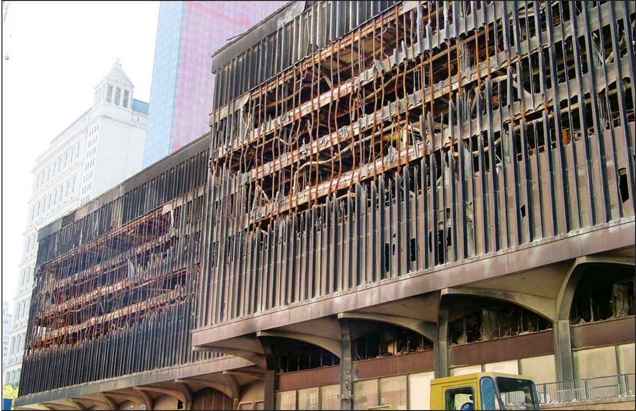
Figure 4-11 WTC 5 façade damage.
