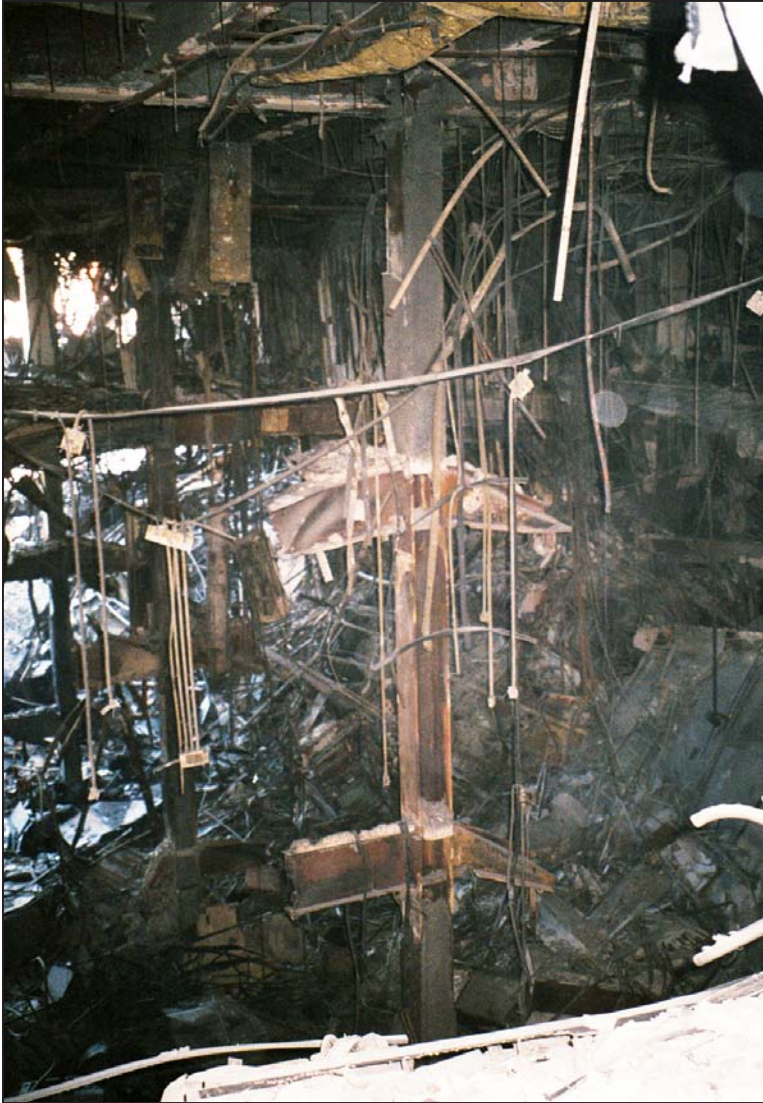
Figure 4-19 Internal collapsed area in WTC 5.
